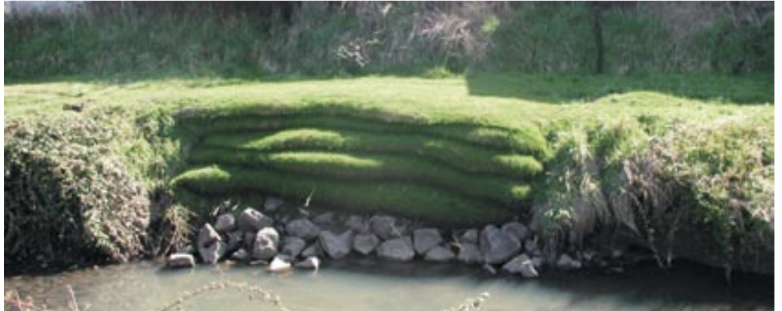
Native willow cuttings, grasses and riparian herbs have sprouted on this repair project between Polk and Garfield Streets, providing slope stability and erosion control.
